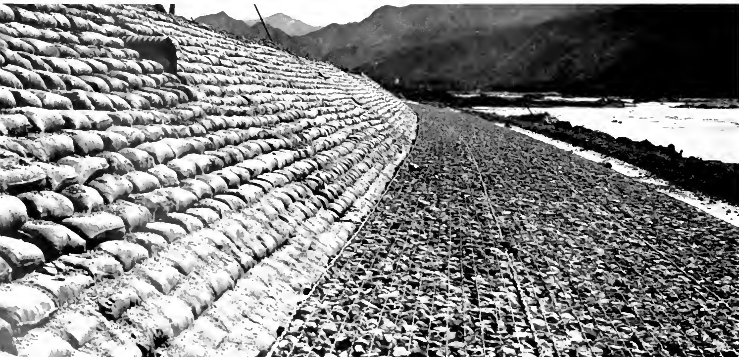
Sacked concrete riprap, 12 inches thick with rock and wire toe mattress, 8 inches thick and 14 feet 6 inches wide
